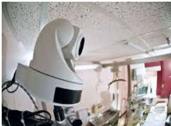
Fig. 1: Wall mounted Wi-Fi IP camera
